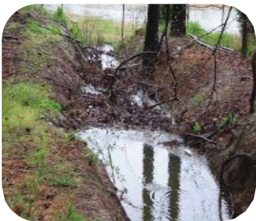
Tree branches and leaves dumped by homeowners are a common cause of storm drain blockages that contribute to flooding during heavy rains.
